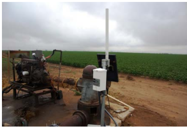
Surface turbine irrigation well
