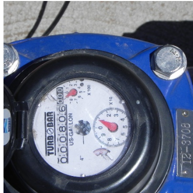
Water meter on system
