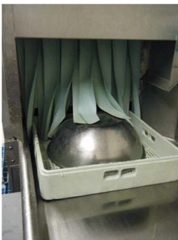
Cafeteria dishwasher, Cedar Park High School, Leander ISD, Cedar Park, Texas
