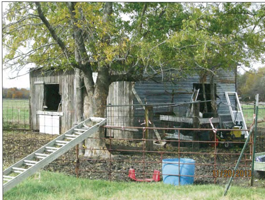
Figure 55. The south and the east walls of the composite shed. Note the three different materials used for construction. View is to the northwest.
