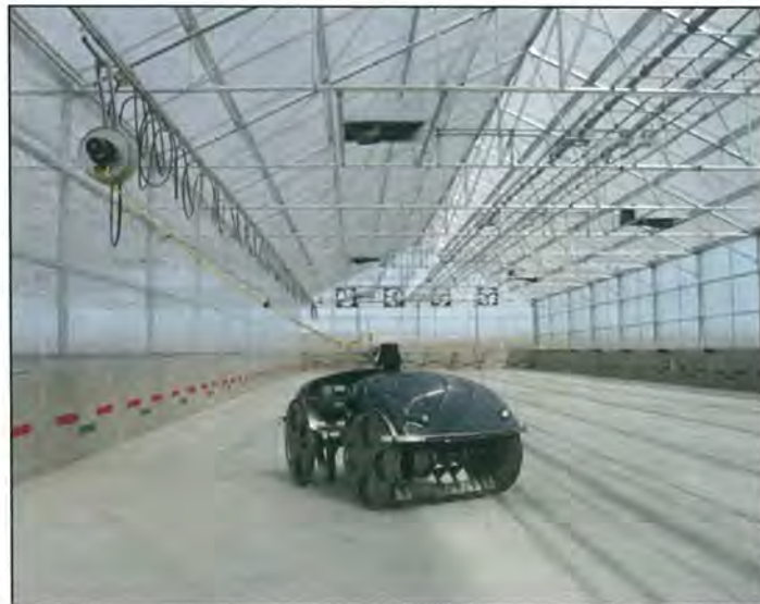
Figure 6: Mole-Type Solar Drying System (courtesy of Parkson)
