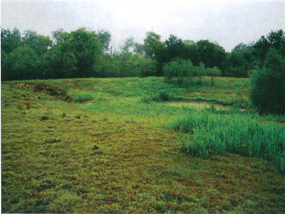
P49. Looking north at WI1. The breach of WI1 is located on the left hand side of the photograph.
