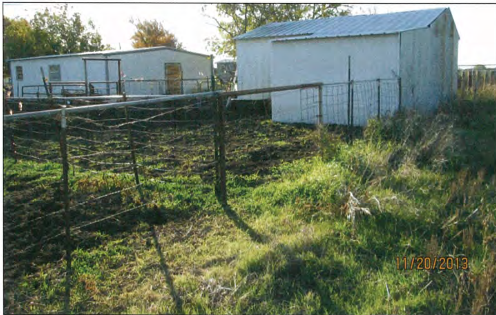
Figure 54. The north and west walls of the composite shed. View is to the southeast.
