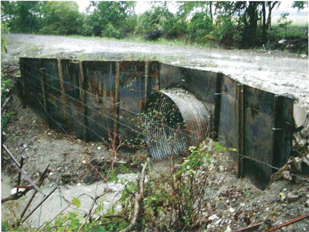
P43. Large diameter pipe culvert beneath County Road 4945 conveying flows for TBC.
