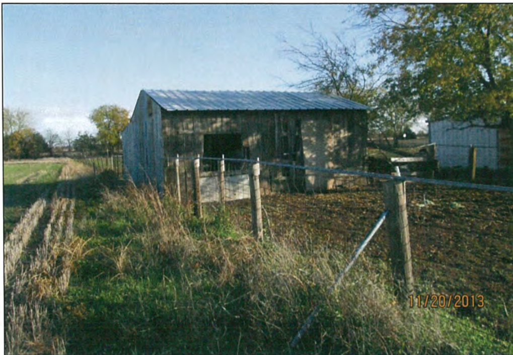
Figure 53. The south and west walls of the composite shed. View is to the northeast.
