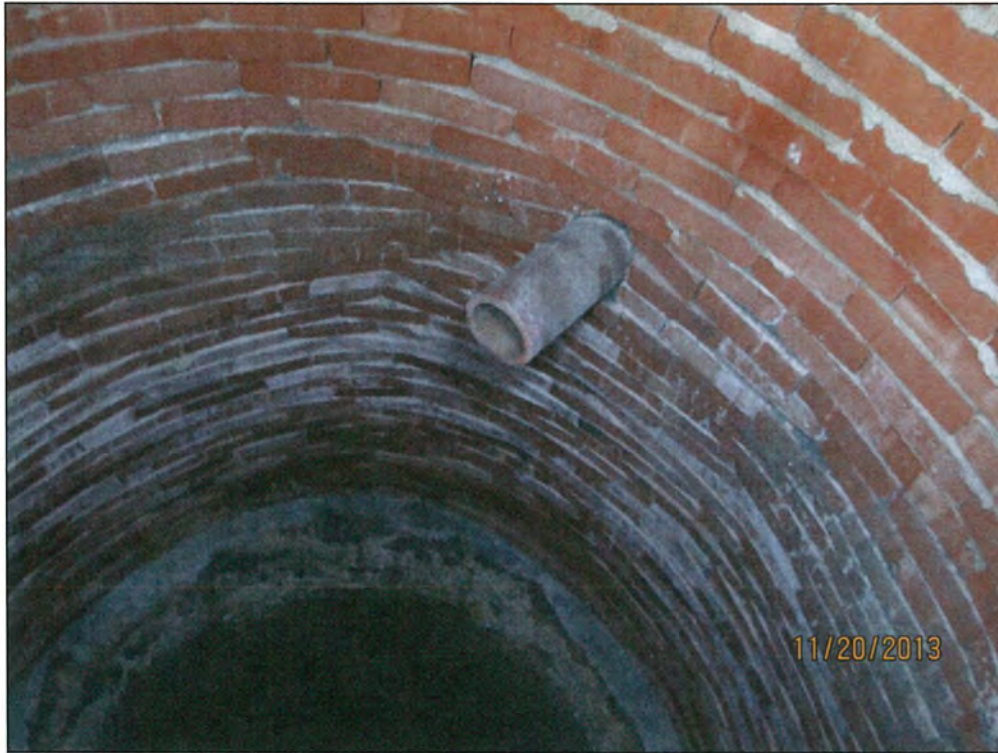
Figure 56. View inside the well-cistern with exposed clay intake line. Note no plaster lining appears to be present.
