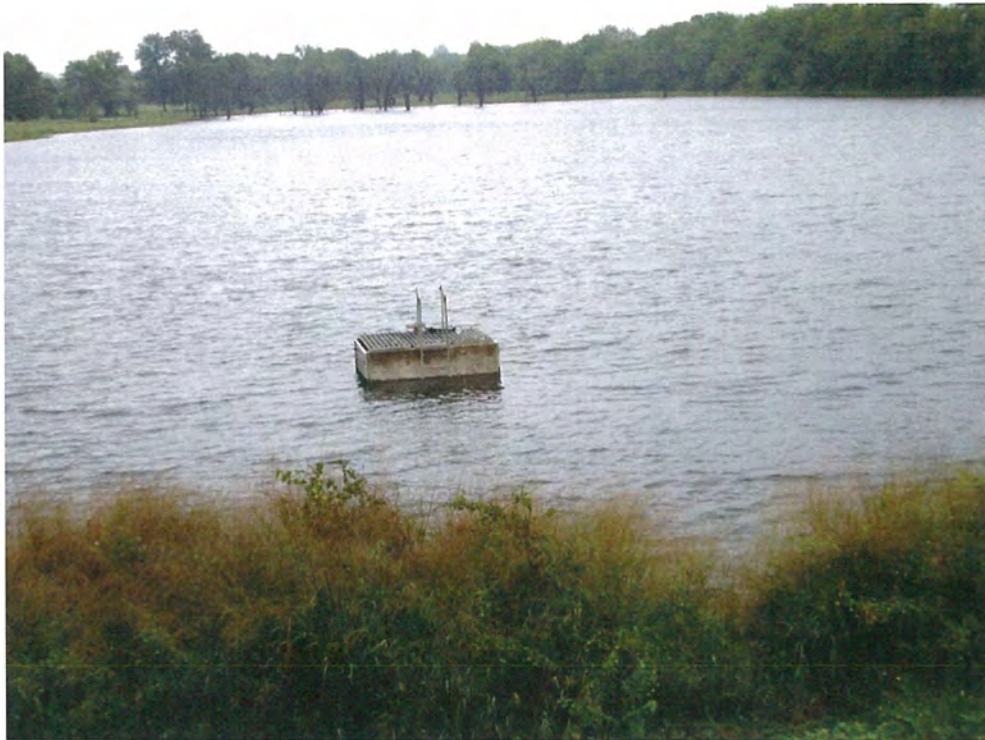
P9. Discharge structure located within the Lee Creek impoundment.
