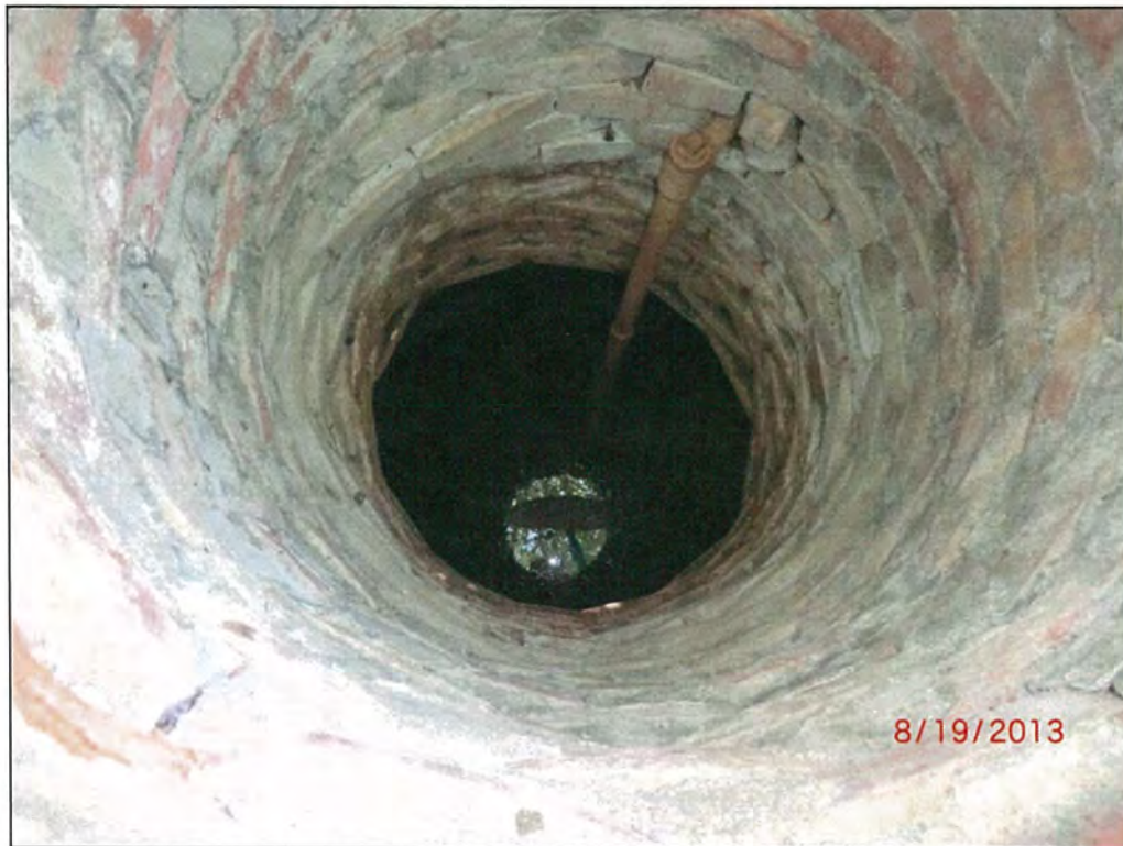
Figure 44. View looking down into the well-cistern at site 41FN170. Note the eroded plaster lining on some of the bricks.
