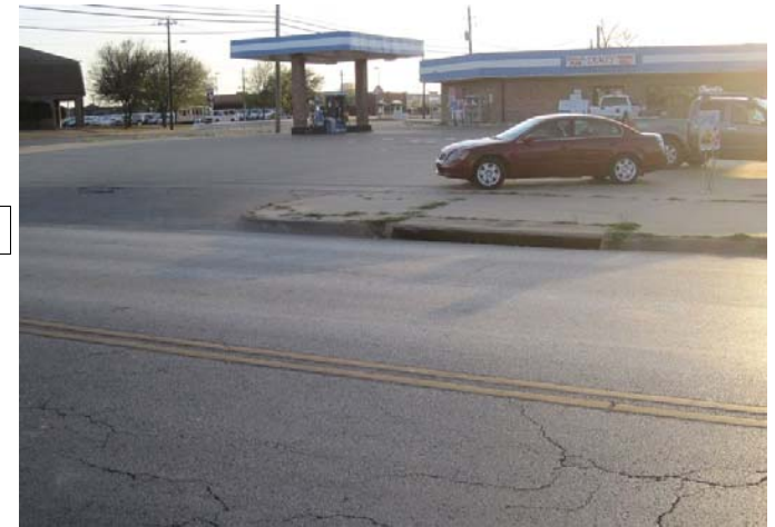
Looking west on Rhea Road at existing inlet south of Covington Dr.
