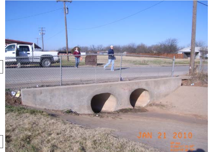
Outfall of East Plum Creek with 2-36" RCPs on the east side of Ridgeway Dr.
