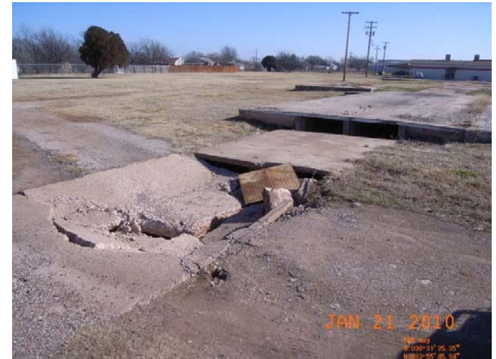
Collapsed box culverts north of Iowa Park Rd.
