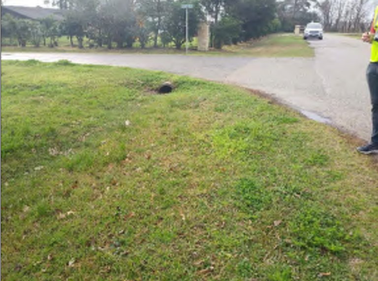
Photo #: 094023 Photo Date: 02/11/19 Location: S Kolbe Drive at Laura Circle Description: Culvert shows 50% silting on east side of roadway. Photo taken looking south towards dead-end.
