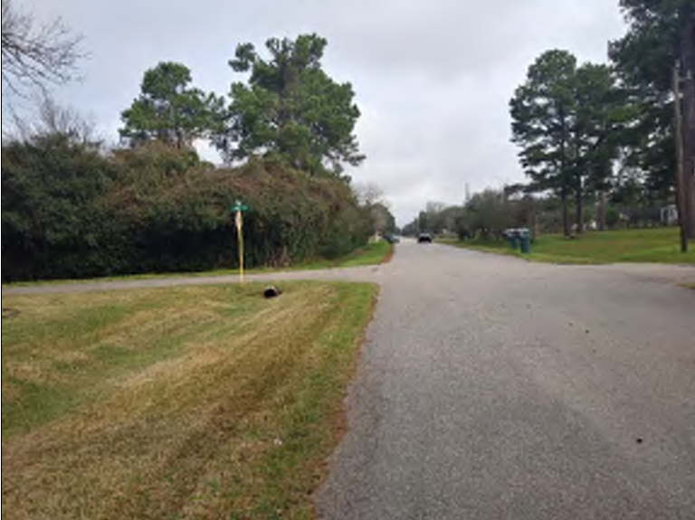
Photo #: 093932 Photo Date: 02/11/19 Location: S Kolbe Drive at Laura Circle Description: Ditch on west side of roadway. No significant silting present.
