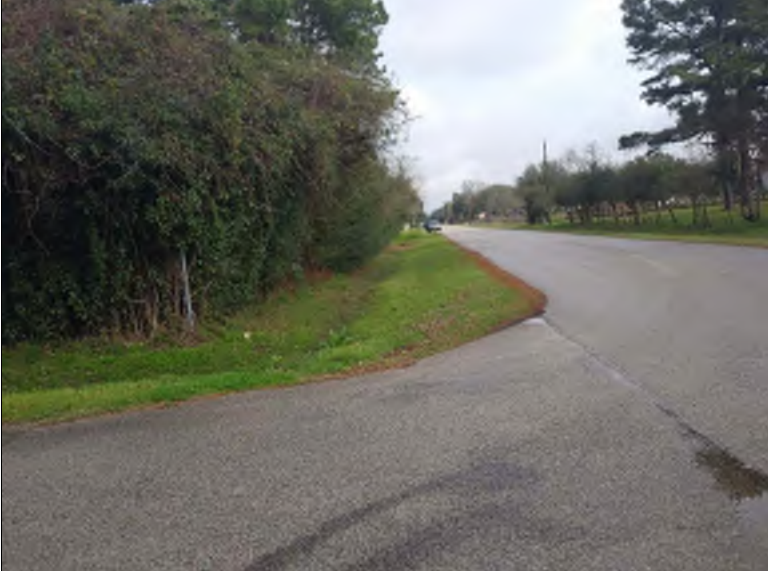
Photo #: 094009 Photo Date: 02/11/19 Location: S Kolbe Drive at Laura Circle Description: Ditch on west side of roadway with steep backslopes.
