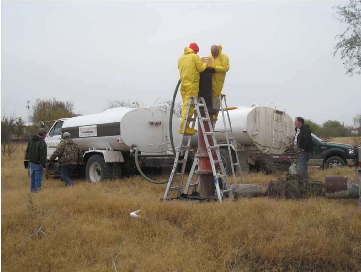
Figure 4.5. Injection of Uranine Dye into Dooley Well on December 17, 2008
