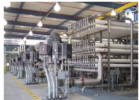
The El Paso-Fort Bliss brackish groundwater desalination facility.
