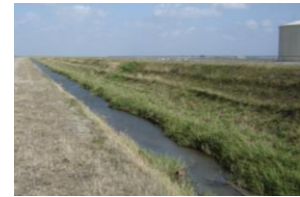
Drainage channel used for discharge of desalination concentrate, North Cameron Regional Water Project, February 2006.
