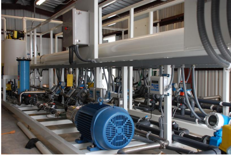
Pilot scale reverse osmosis skid, Brownsville Seawater Desalination Project, Texas. Photograph courtesy of NRS Consulting Engineers
