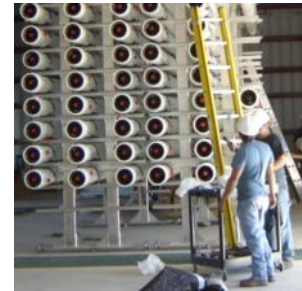
Assembly of the pressure vessel racks, North Cameron Regional Water Project, December 2005.
