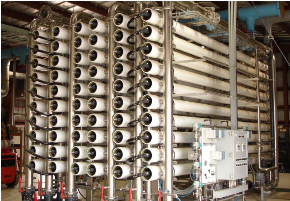
Reverse osmosis membrane array, North Cameron Regional Water Project.
