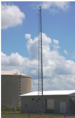
Communications tower for the supervisory control and data acquisition system, North Cameron Regional Water Project, August 2007.
