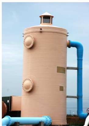
Degasifier, North Cameron Regional Water Project, June 2007.
