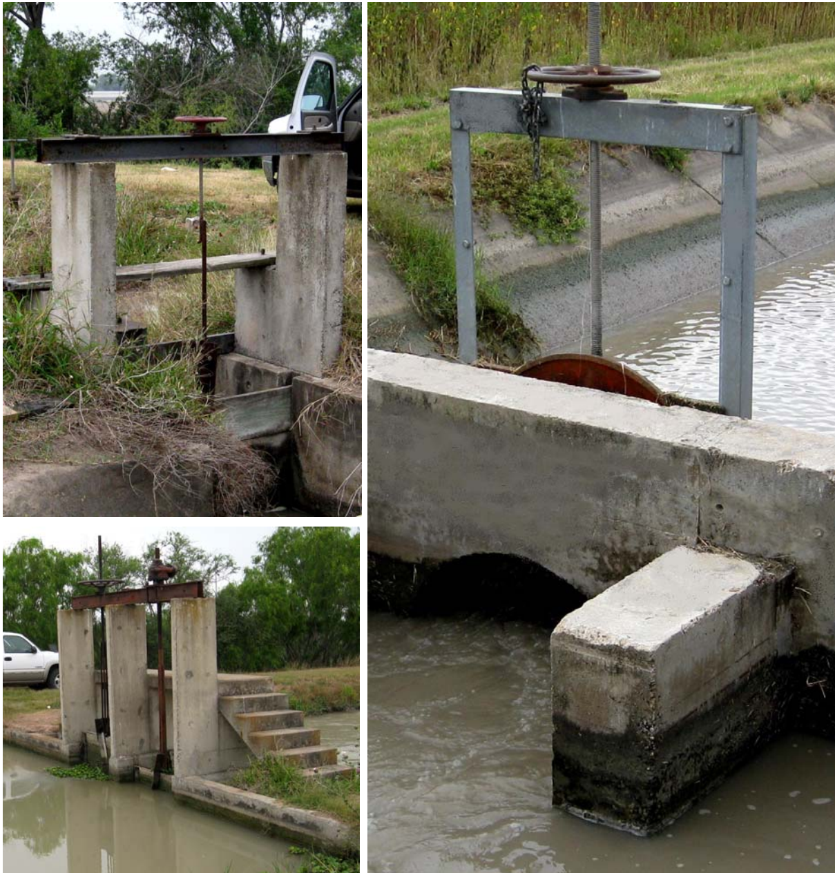
Figure 1. Various manual gates requiring an operator to raise and lower them.
