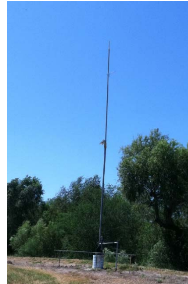
Figure 2 LCRTU and Extended Antenna
