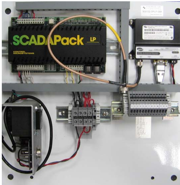
Figure 16. A SCADA system capable of automating gate operation in response to input from a sensor such as water level.
