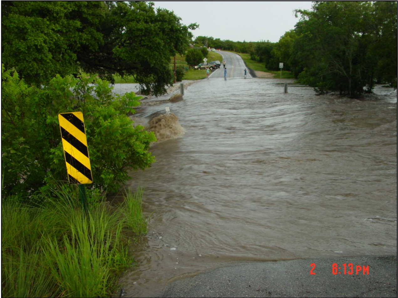
Figure 2: McGregor Lane overtopping during 2007 event
