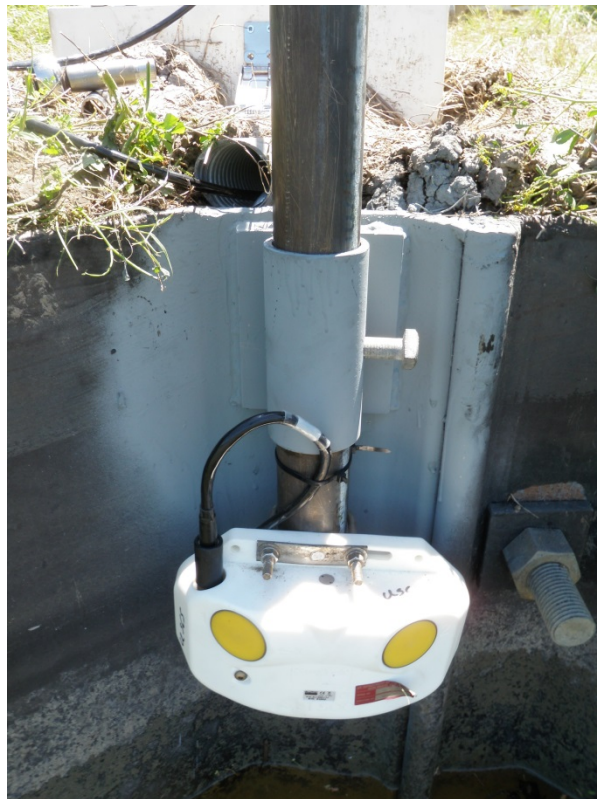
Figure 2. Sontek Argonaut SL 1500 installed at USGS streamflow gaging station 08067252 Trinity River at Wallisville, Tex
