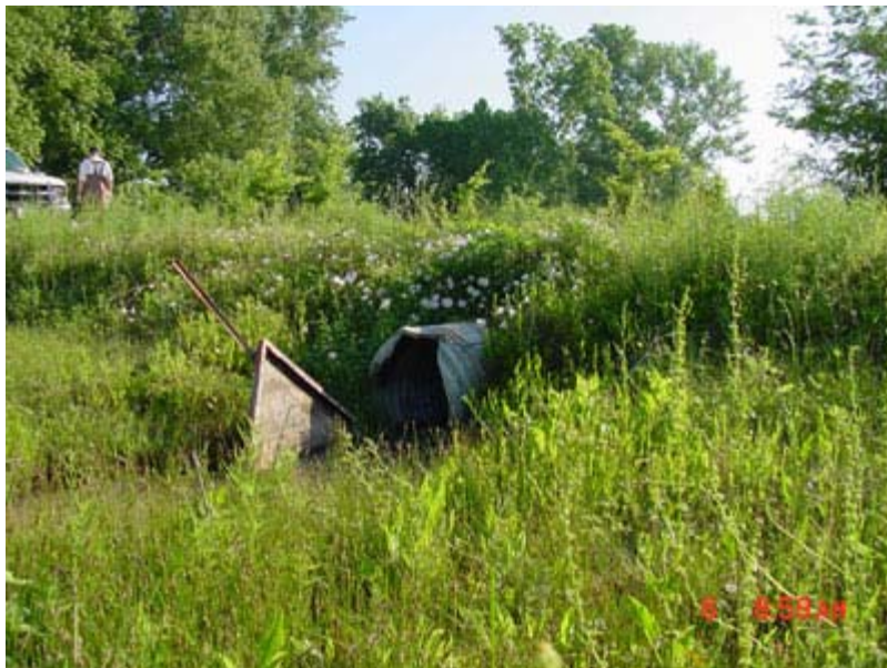
Figure 3.5 – One of two cylindrical culverts running through the road embankment. These culverts will transmit water from the Brazos River to Moelhman Slough at river stages lower than the reported control elevation, but the volume of water transmitted is too small to consider the river and slough as “connected”.
