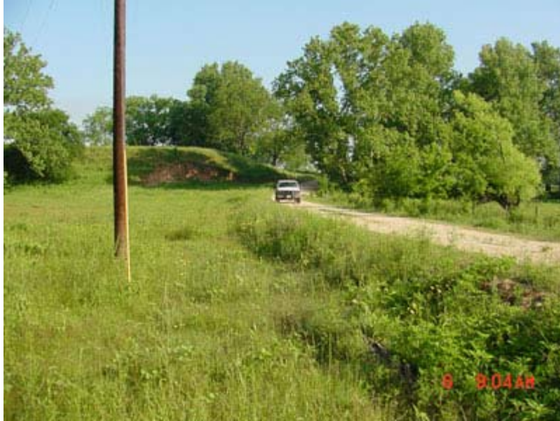
Figure 3.4 – Dirt Road Embankment crossing the old river channel between Moelhman Slough and the Brazos River. The flow channel shown in Figure 3.3 is off to the right of the view shown here.
