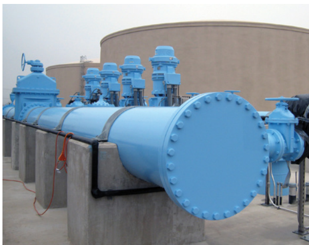
A pump station as part of a TWDB-funded water supply project
